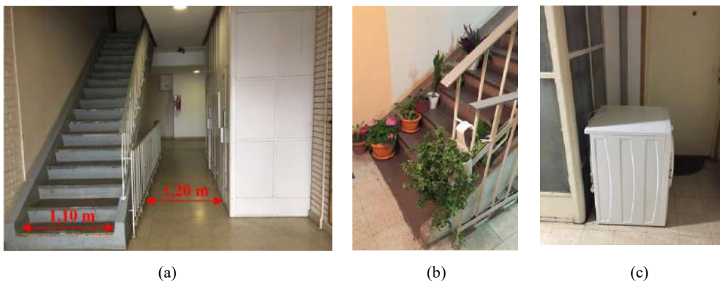
Figure 8 – Evacuation routes: (a) insufficient width of the main staircase and hallways; (b) obstacles in the form of potted plants; (c) obstacles in the form of furniture;
